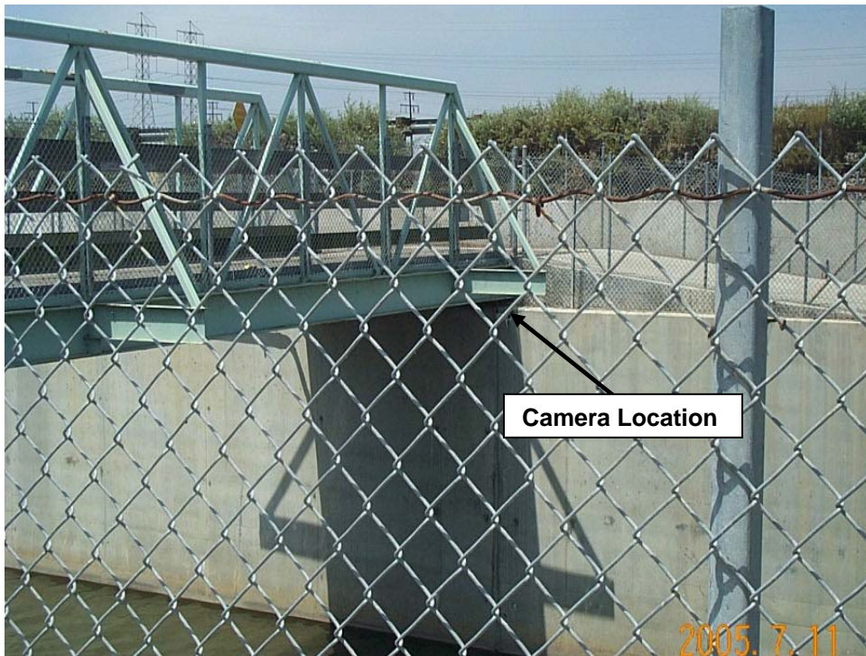
Figure 4 View of Camera Location Installed at Pedestrian Bridge and Channel Wall
