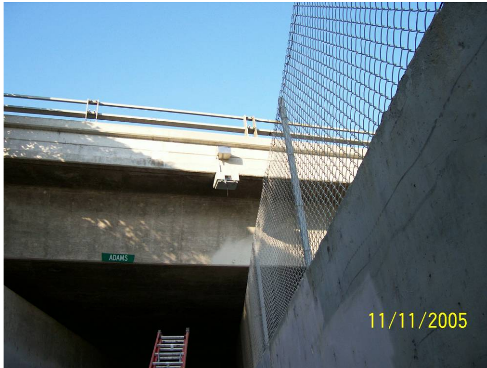
Figure 5 Camera Installation at Adams Avenue Bridge
