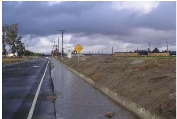
during storm event of December 12, 2009
