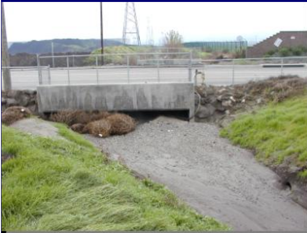
Dirt channel on Kimball Ave (S10)
